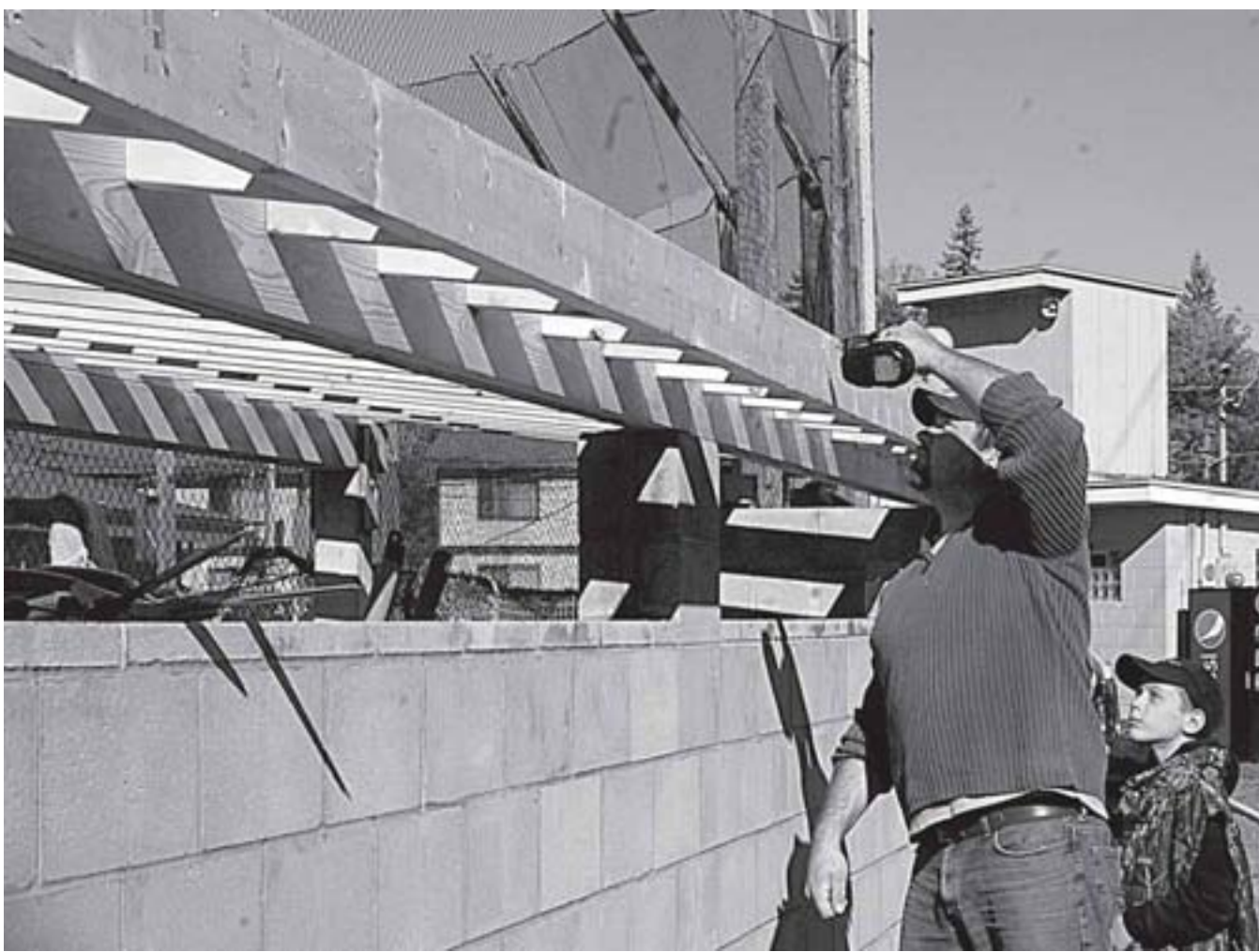
With help from his son Colton, Tim Sisson works on the roof of a dugout at Cobleskill's Little League field on Saturday. The Sissons were among several who were volunteering to rehab the field and dugouts.
