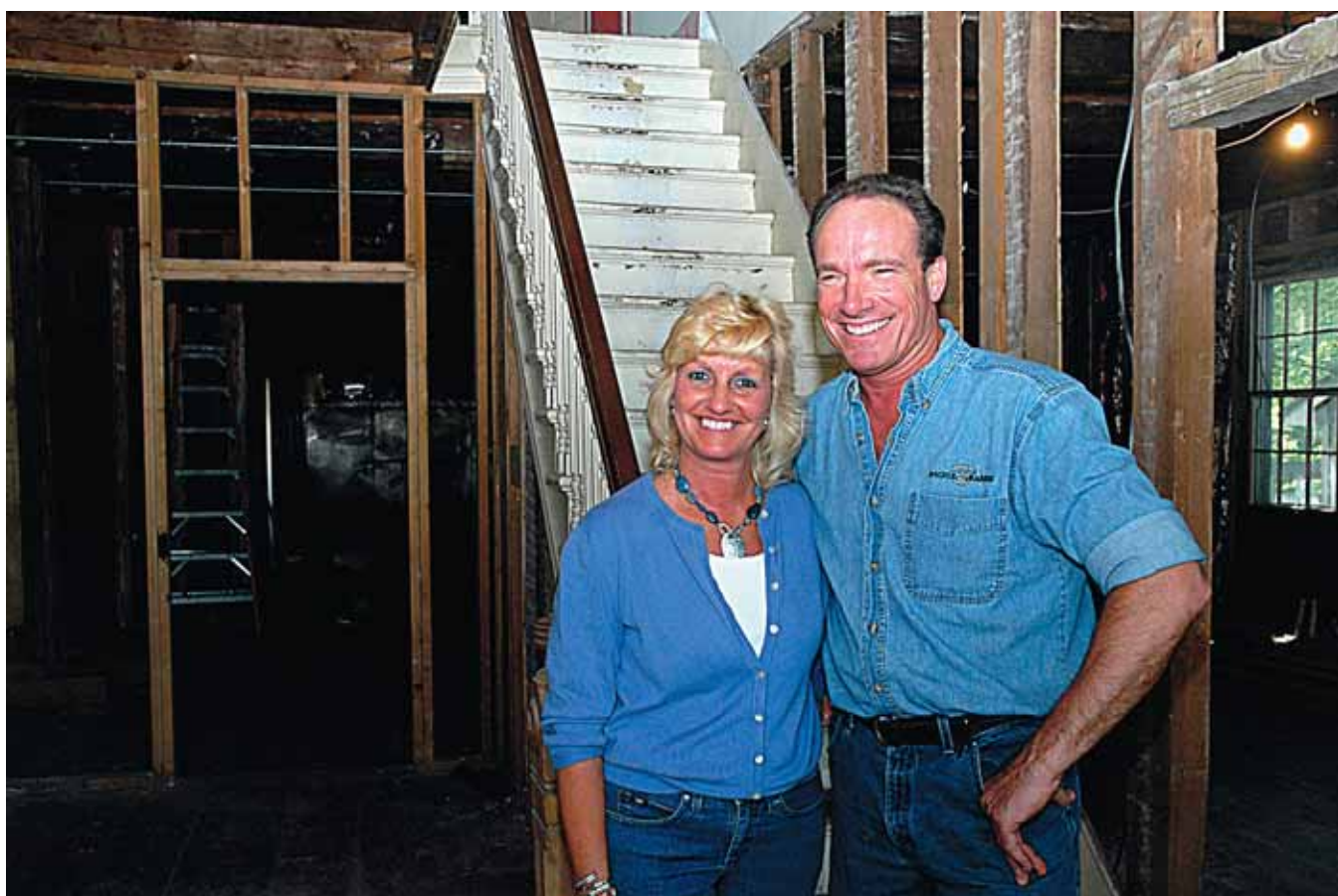
Even though the project is far more than they expected, partners Mary Sagendorf and Chris Guldner are still smiling as they stand in their gutted Bull's Head Inn on Friday. They originally expected to open the historic inn in late summer. Now they're eying an end-of-year opening day.
